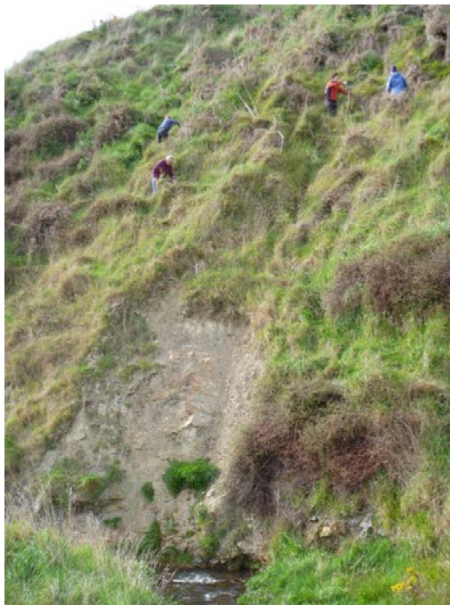
Bluff and slip above Whareroa Stream
