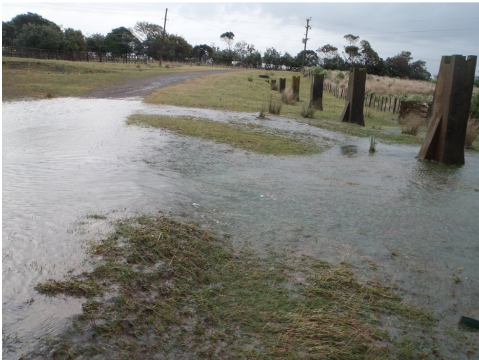
The culvert under the main race blocked
