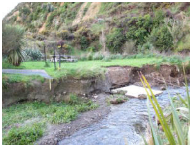
Concrete slab fell into stream in Sept
