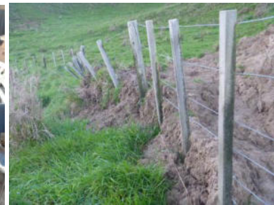
Slip above the Cairn damaged fencing
