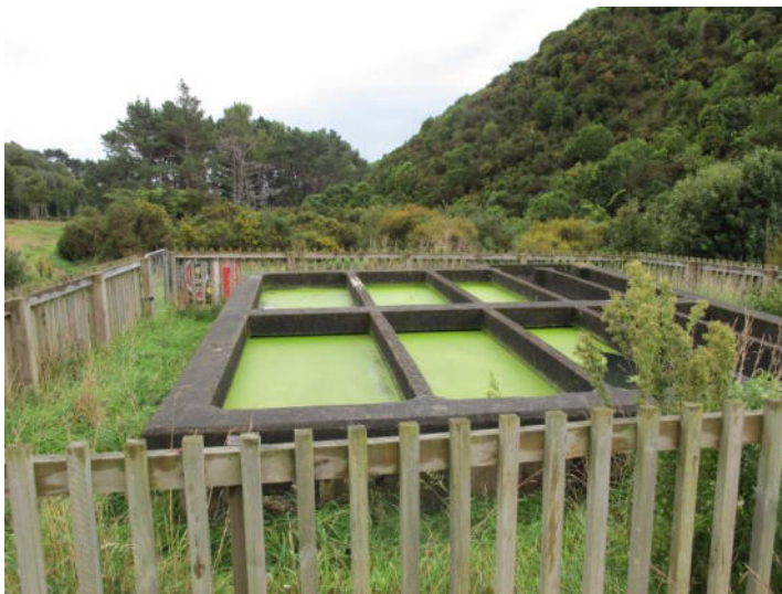
Water Intake settlement chamber, full after heavy rain
