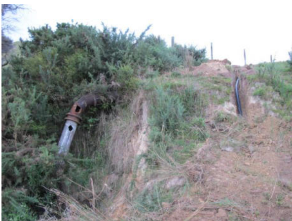
Old pipe to left, new pipe to right, going up to reservoir
