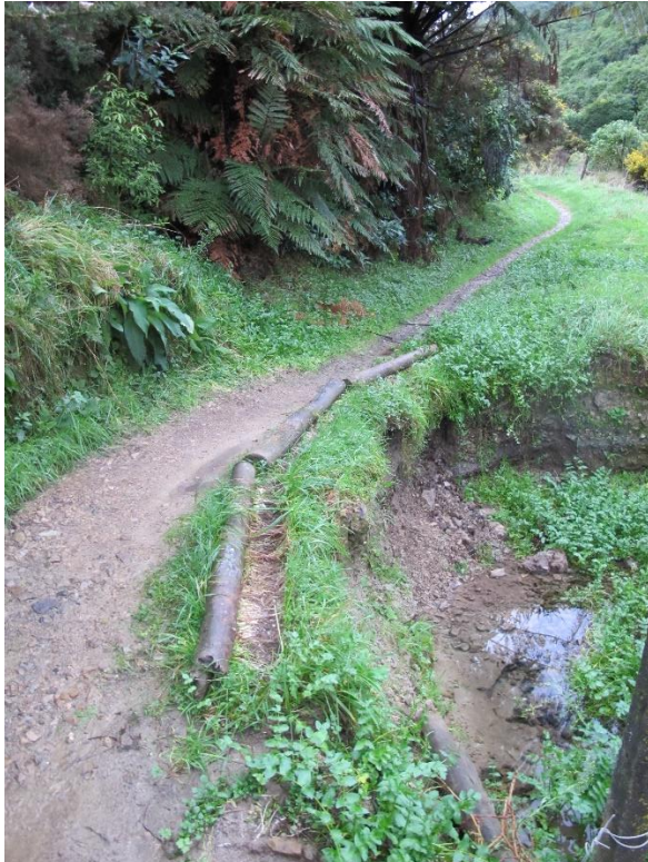
Undercutting of Link Track
